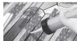
REPLACE CAULKING IN AREAS WHERE NEEDED WITH TEAK JAMMER
